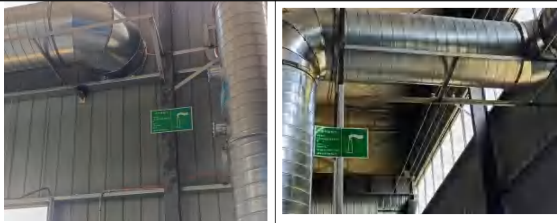
颗粒物废气排气筒 DA001、有机废气排气筒 DA002
